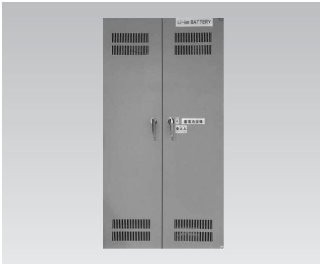
Fig. 3: A photo of the lithium ion battery panel
